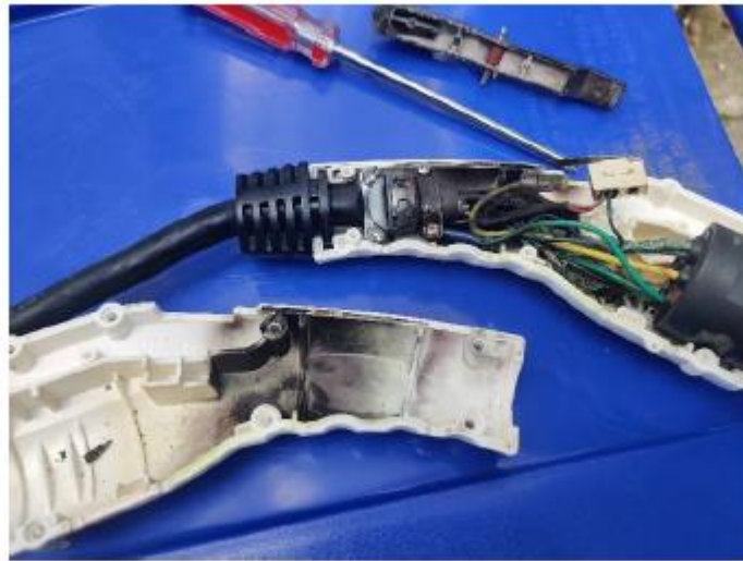
Figure 3. Inspection of a connector producing smoke during a charge session [6].
